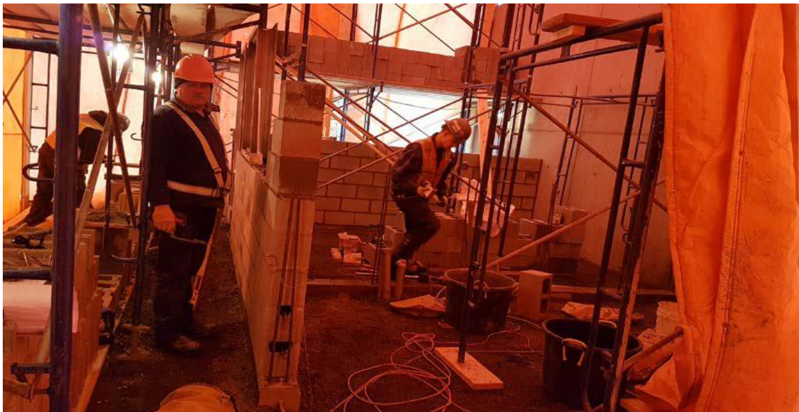
Masonry walls started in front of the building in heated covered space.
