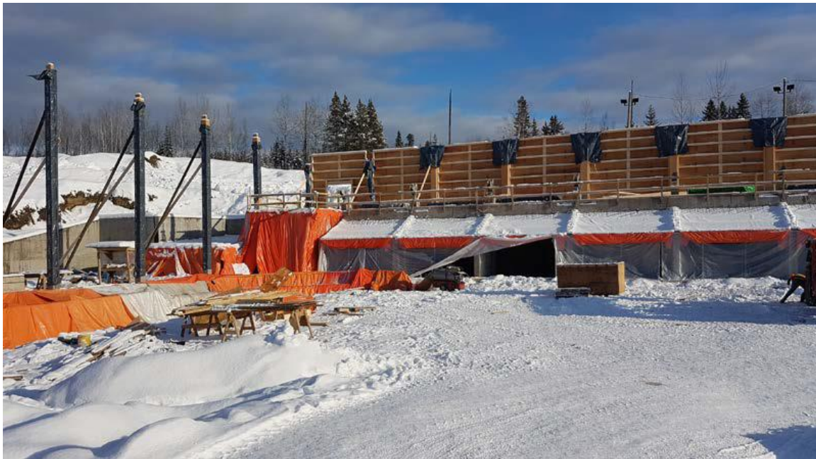
Photo 2 - Wall panels and glulam columns ongoing, also header trench ready to be poured
