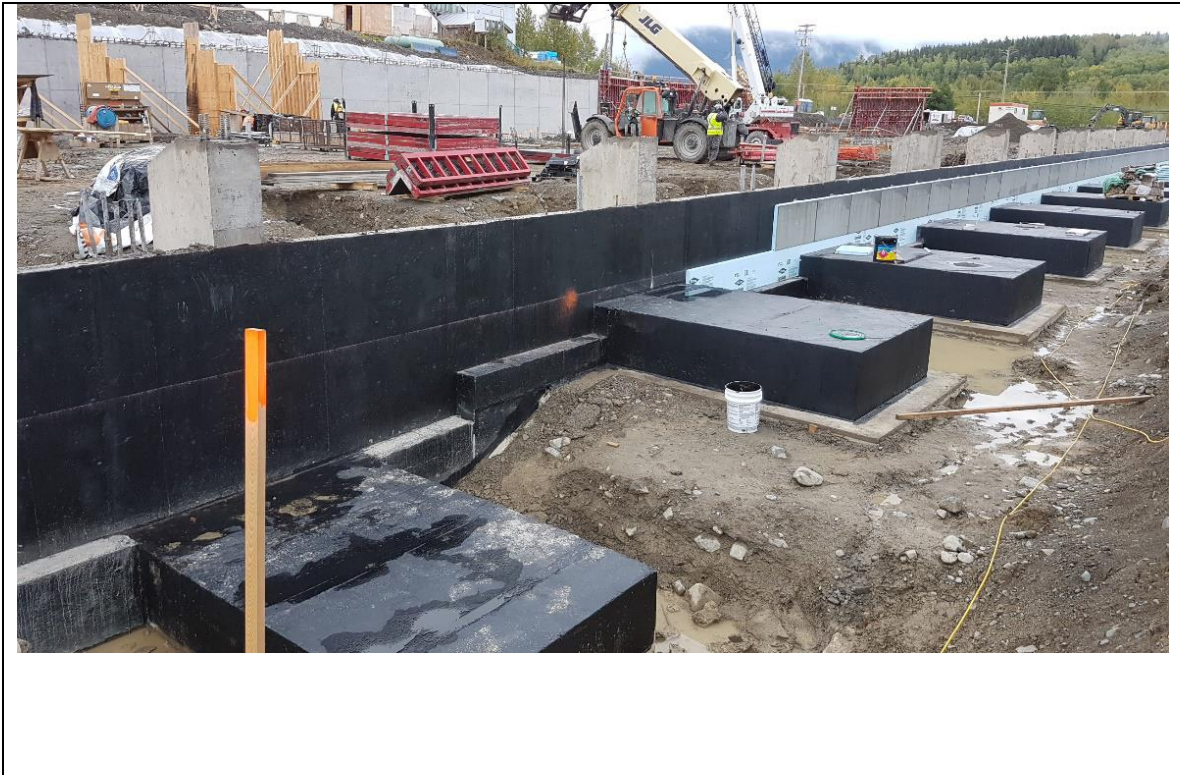
Concrete Support Footings for Structural Beams, Exterior Wall Damp proofing and Insulation
